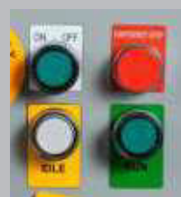
Control panel labelling
