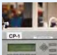
Control panel and electrical panel labels
