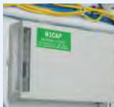
Control panel labelling
